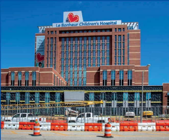
The four-floor hospital expansion includes 128,575 square feet of total construction with more than 104,000 square feet of new construction.
