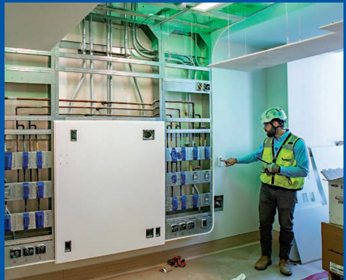
Turner Construction senior project manager, Blake Tyler, demonstrates state-of-the-art features in the new CVICU room, including a special ceiling constellation panel that patients can change from their bed.
